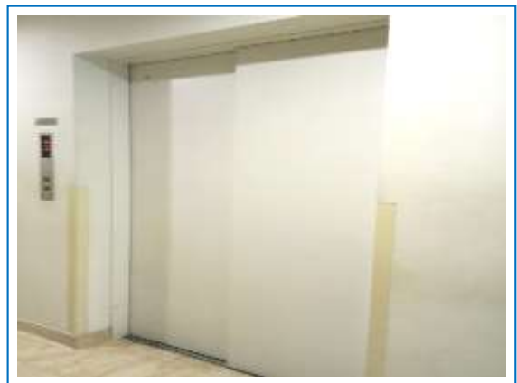
Lift barang lantai 20
